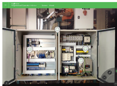
Virtually-open electrical cabinet
