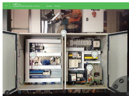
Virtually-open electrical cabinet
