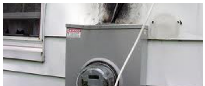
Service entrance destroyed by a surge
