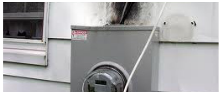
Service entrance destroyed by a surge
