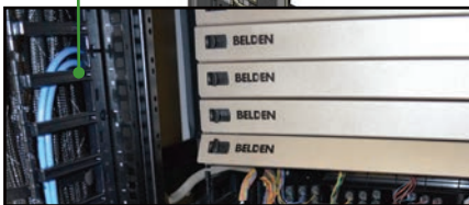
Vertical Manager shown in cabinet
