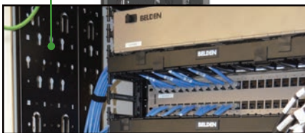
Lacing Panel shown in cabinet
