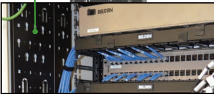
Lacing Panel shown in cabinet
