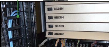
Vertical Manager shown in cabinet
