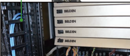
Vertical Manager shown in cabinet
