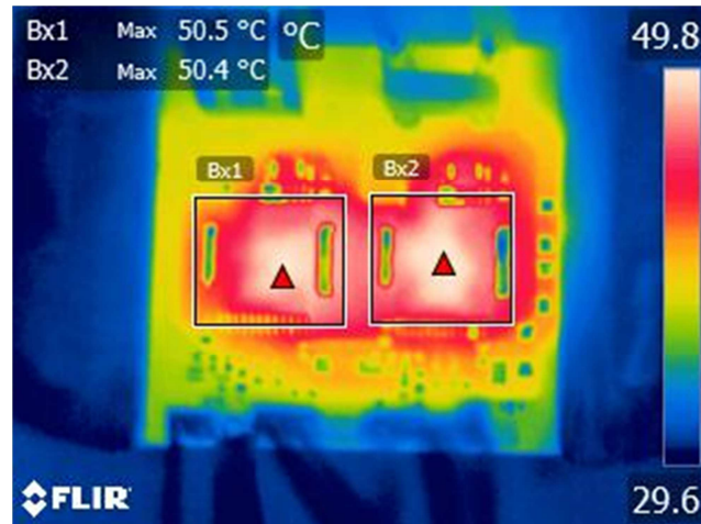
Figure 19 – Thermal Scan at 15 W Inverter Output in Self-Supply Operation.
